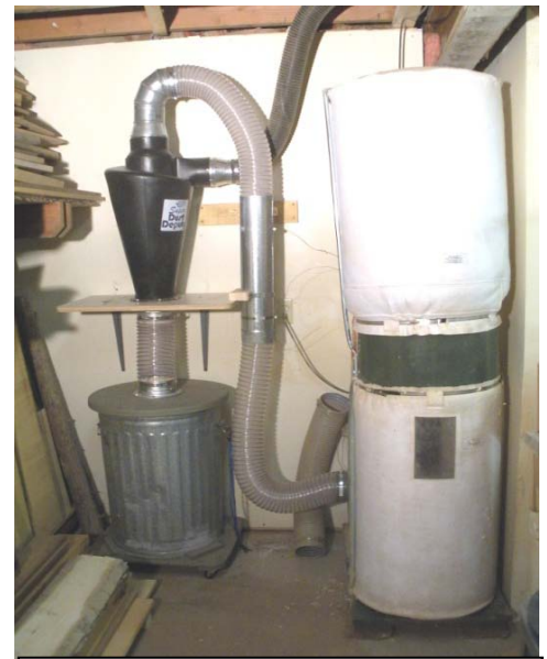
Completed installation of the Super Dust Deputy showing connections to existing system.
